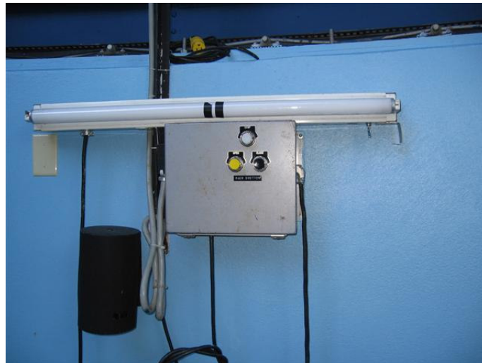
Figure 6: Dome shutter control panel with pushbutton switches to open and close the shutter.
