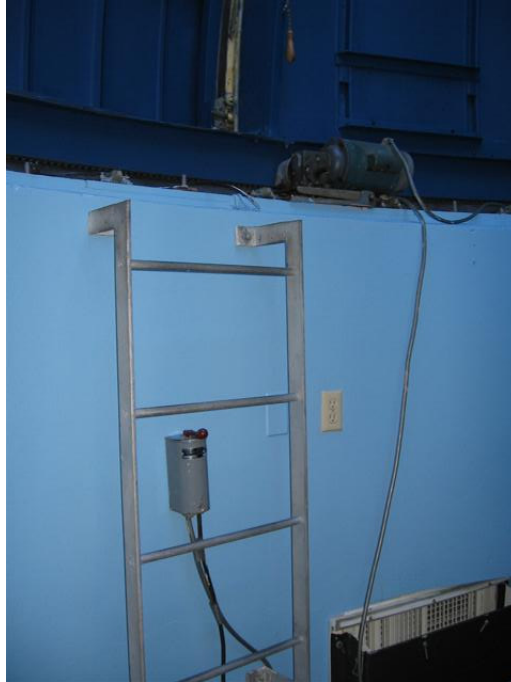
Figure 7: Dome motor control switch and ladder. Note the west dome motor in upper right of photo.
